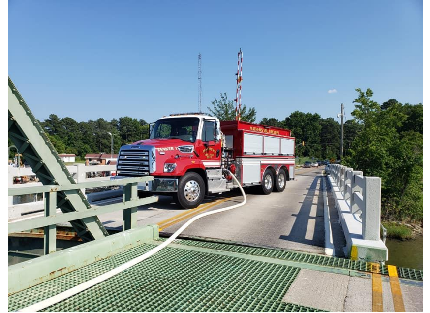
Residents have been delayed during days of extreme temperature when expanded steel prevents the bridge's swing span from closing. The Mathews Volunteer Fire Department assisted during this June 2020 incident by pumping water on the bridge to cool the steel. Photo credit: Mathews Volunteer Fire Department
