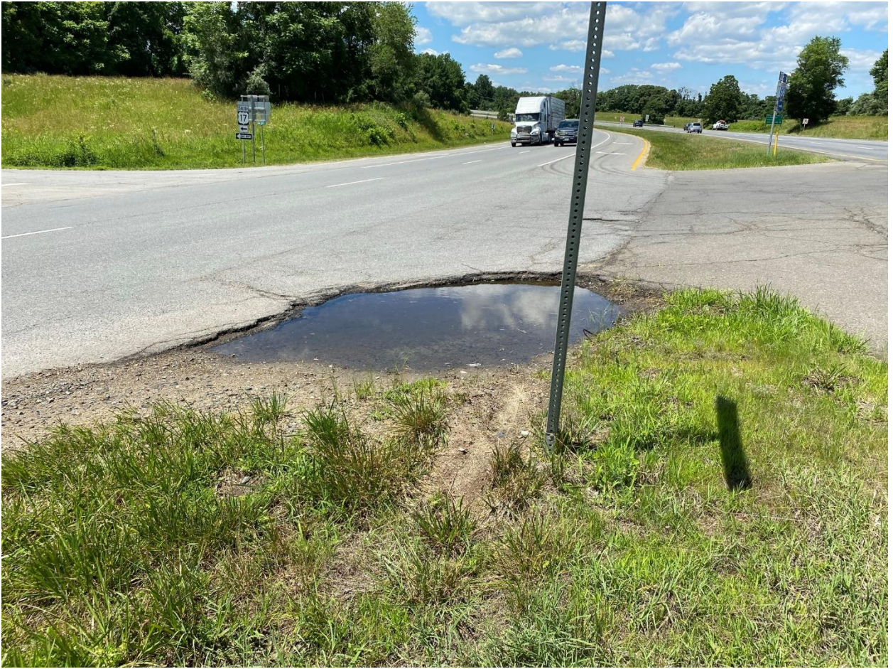
Figure A.10 Damaged pavement on the median opening area
