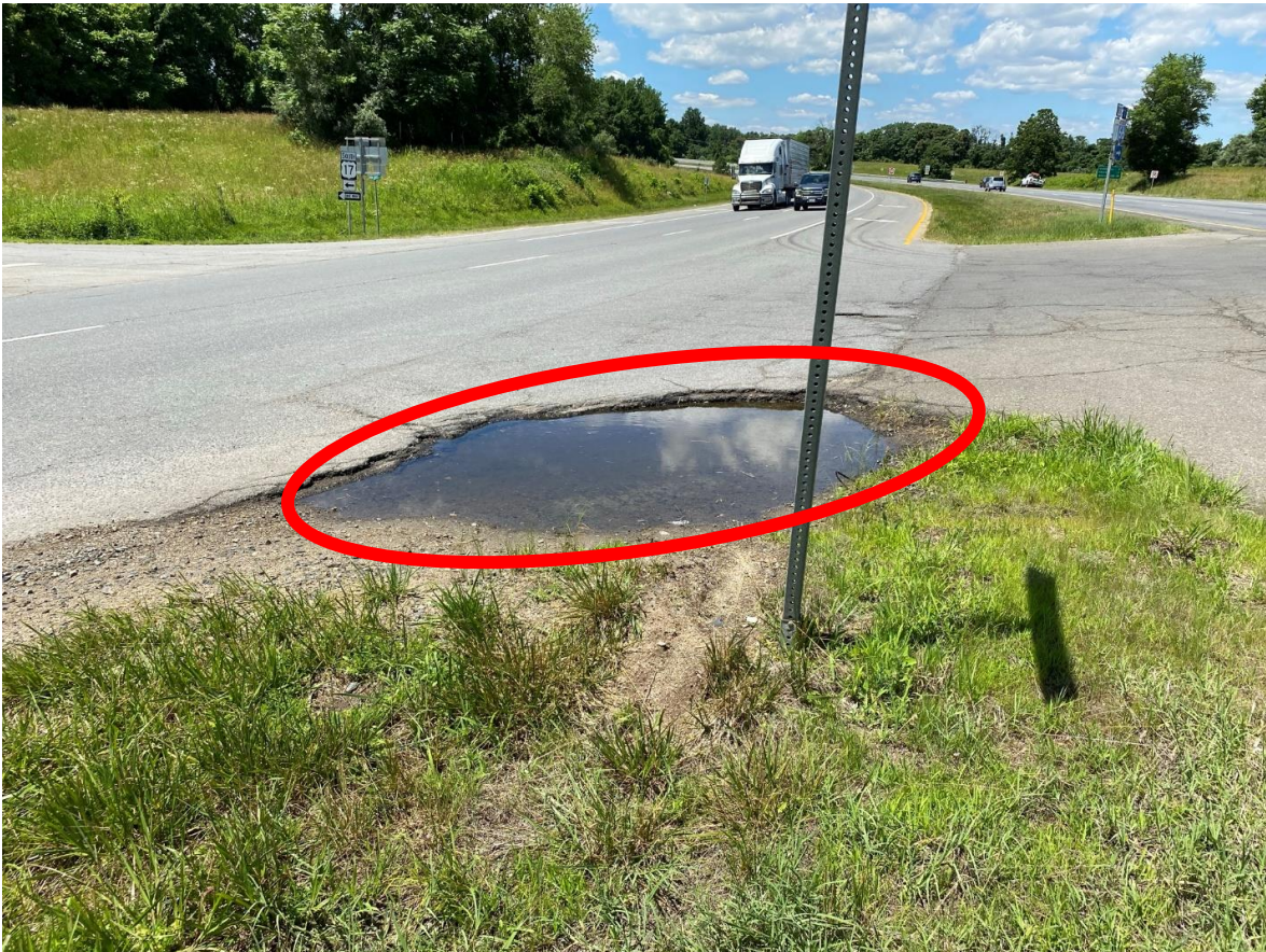
Figure 2. Damaged pavement to be repaired
