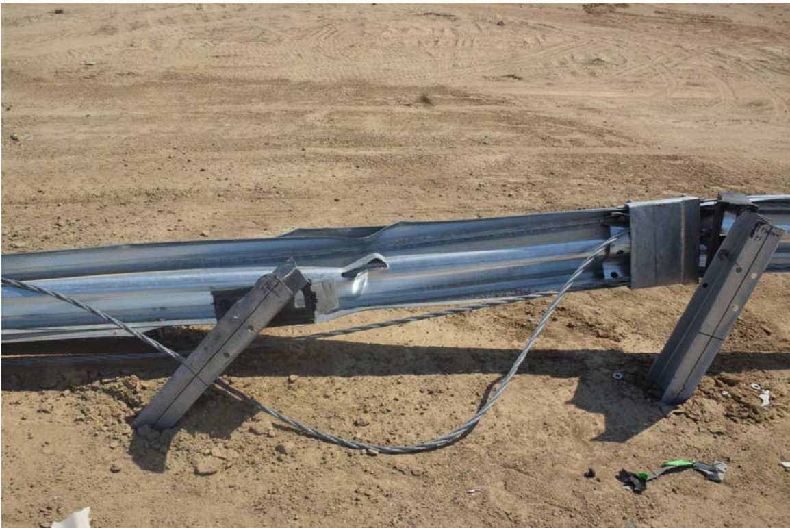
FIGURE 40. Test Article Damage
