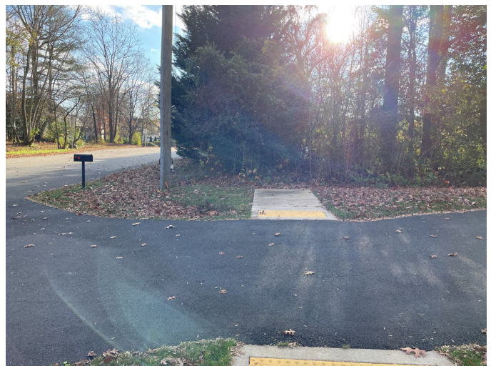
Figure 31: Sidewalk gap on Old Burke Lake Road.
